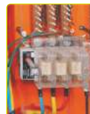
(SFU) Switch Fuse Unit
